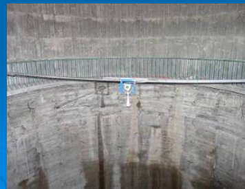
Measurement of surge tank water levels by radar.
