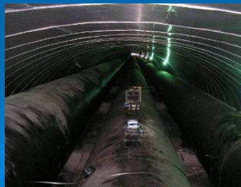
Penstock discharge measurement point.
