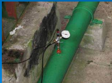
Pressure measurement at upstream end of penstock.
